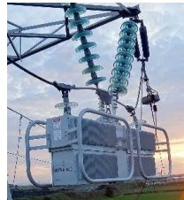
Smart valve load balancing transformer
