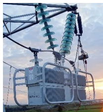
Smart valve load balancing transformer
