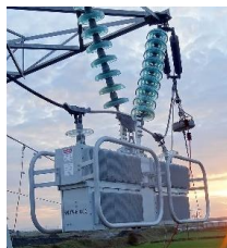
Smart valve load balancing transformer
